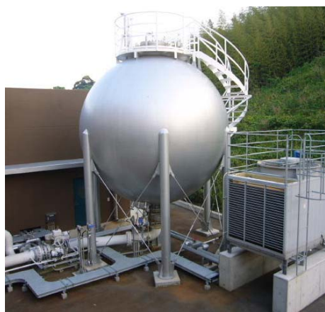
高圧貯気槽 Air Storage Tank, 2.79 MPa
